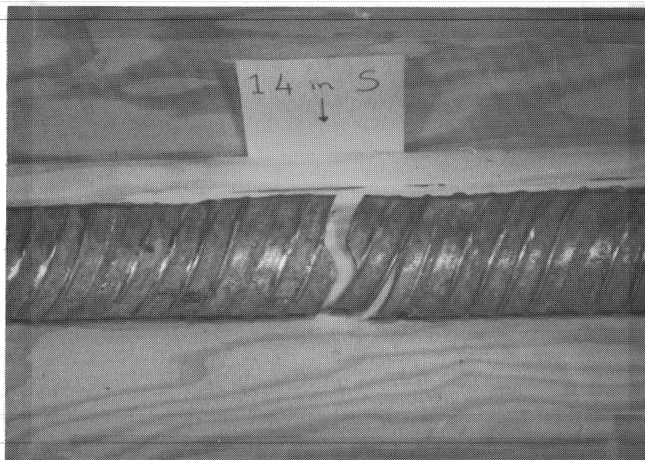
Figure 4.10 Photographs of Fractured Metal Duct
